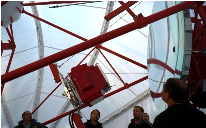
Figure 3: Installation of the GCT camera on the telescope with the Camera Removal Mechanism. The arm is here at an intermediate position between the ground level and the focal surface in front of the secondary mirror visible on the right of the picture ©'The GCT subconsortium'.
